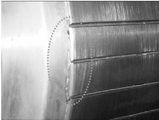
Fig. 11 Suspected cracked or broken area between rotor bar and end-ring
